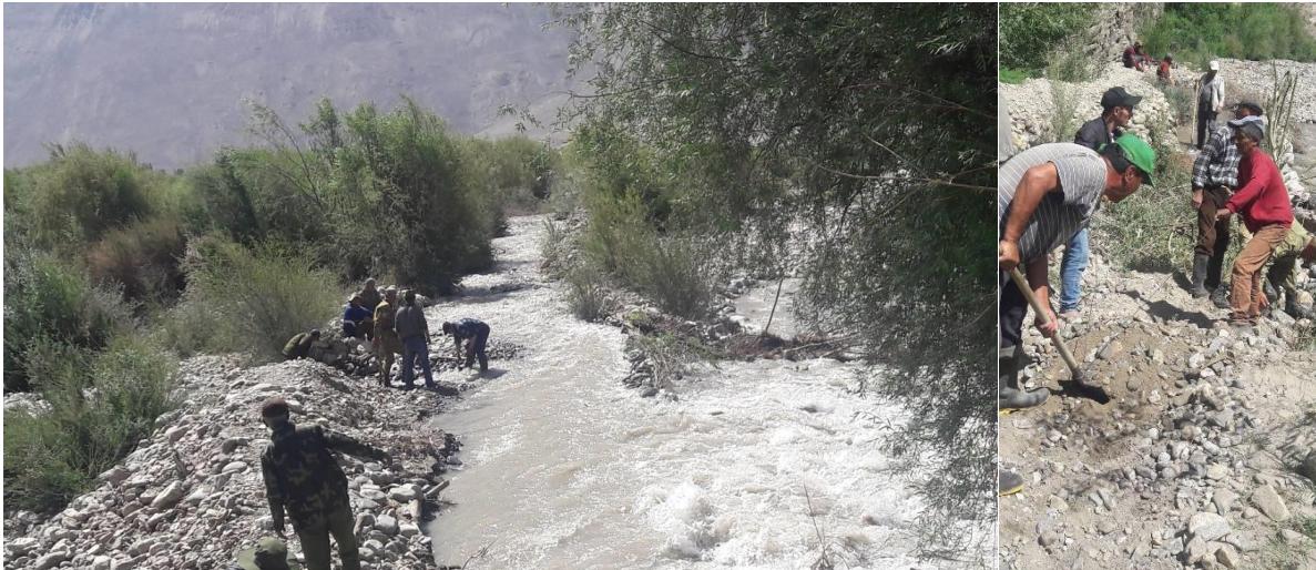
Figure 16. Forest users of Shitkharv village reconstructing the head channel that was destroyed after river flooding. (Photos: U. Khairulloev, 1 August 2019).
