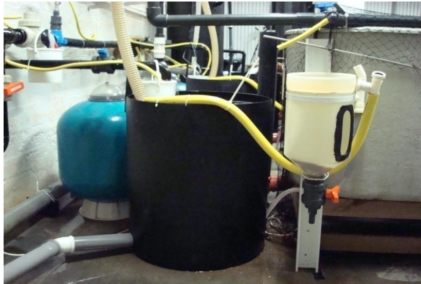
(a) Sedimentation tank
