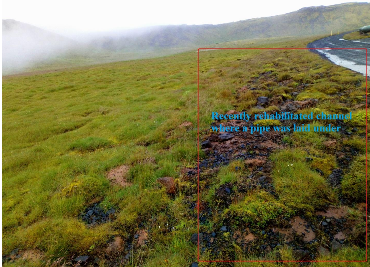
Figure 5. Channel recently rehabilitated using turf transplant at ON Power's site where a pipe was laid out as indicated in the red rectangle.
