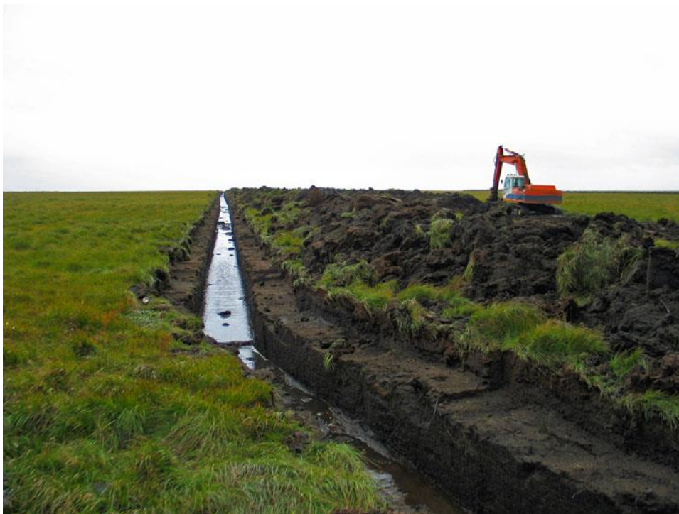
Figure 5: Example of drainage ditch in a wetland of South Iceland (source: http://www.springer.com/us/book/9789401796200 )
