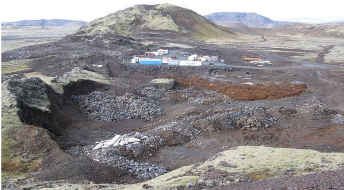
Figure 3. The crater at Gígahnjúkur was first filled with rock and soil materials to replace the rock materials which had been excavated from it (Photo: Námur.is, 2017)
