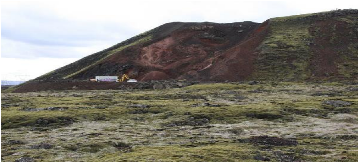
Figure 2. Construction works at Hellisheiði for the geothermal power plant left a large crater at Gígahnjúkur (Photo: Námur.is, 2017)
