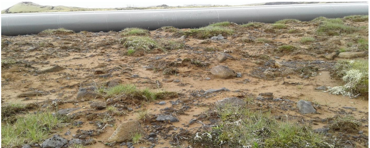
Figure 7. A site at Hellisheiði which had been disturbed through installation of thermal pipes. Here turf transplants have been spread to restore the vegetation of the site (Photo: Emmanuel Mwathunga)
