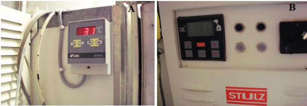
Figure 20: Temperature (A) and relative humidity (B) control panels of storage chamber
