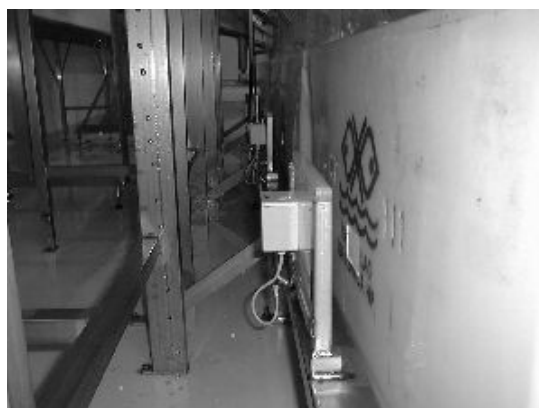
Figure 25: Installation of the electronic reading device (H-039).
