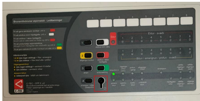
Figure 12 Fire alarm panel.
